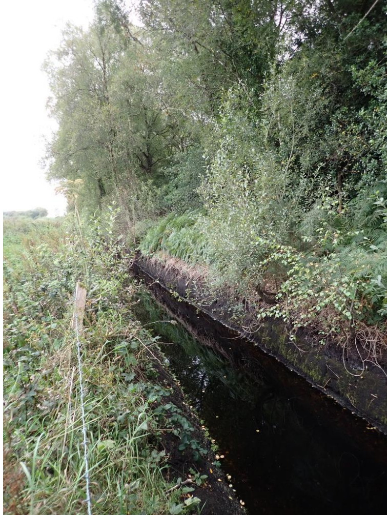
Figure 7 - Typical existing drain cut into peat at the site (photo taken between Turbine 8 and 9 and intended to show a typical existing feature, not future construction)
